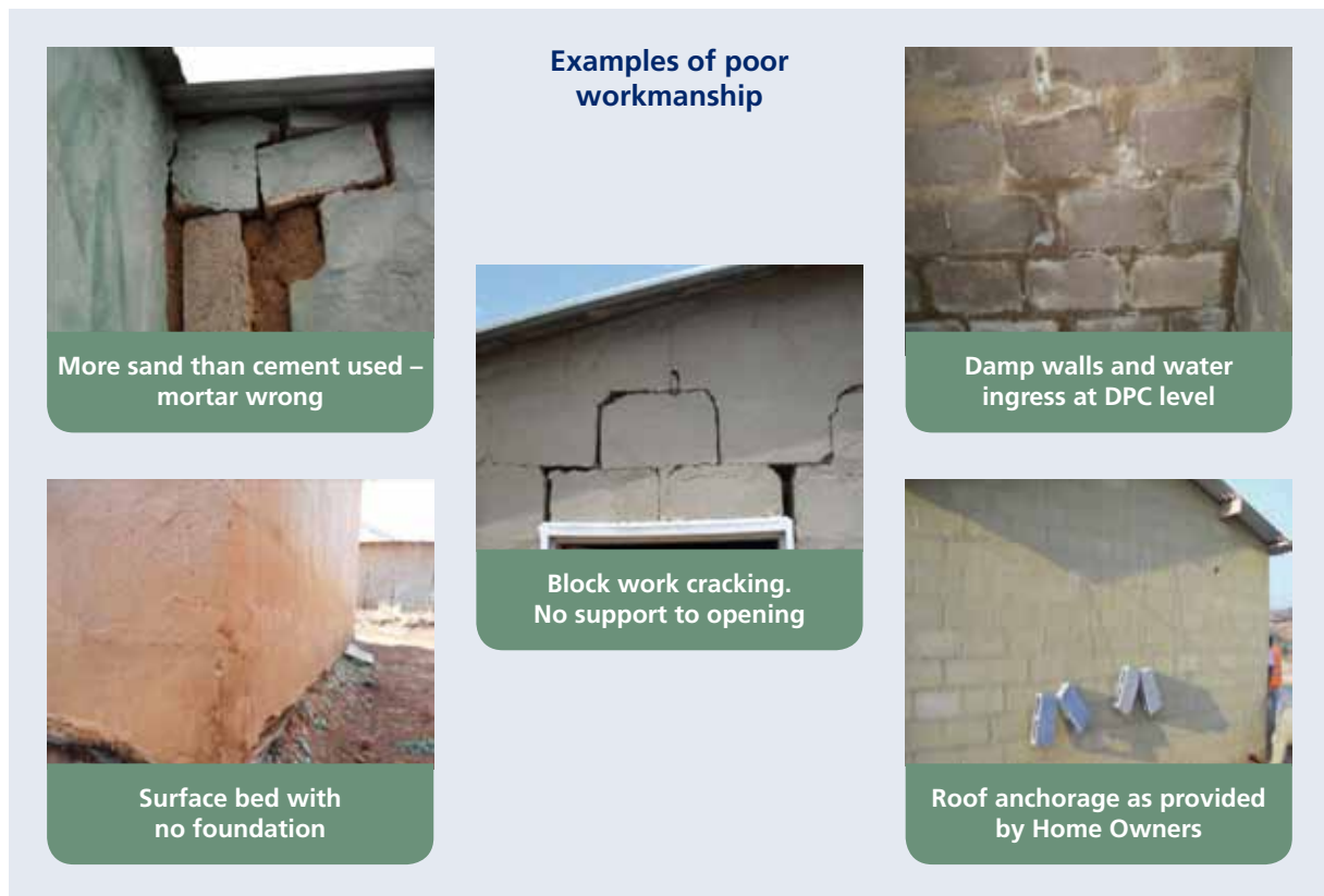
Figure 13: Examples of defects found in houses
