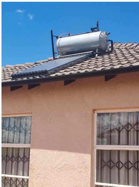
Figure 29: Front view of solar geyser
