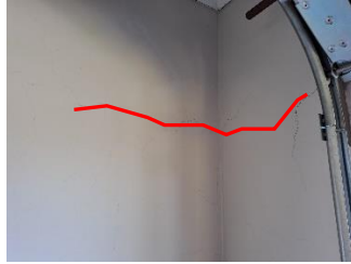
Pic 09: Diagonal crack on both walls joining at the corner
