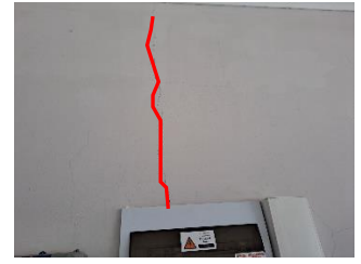
Pic 11: Vertical crack above DB board in the garage
