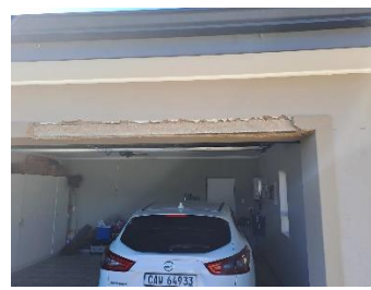
Pic 06: Crack above lintel result in plaster band coming loose
