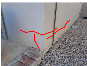
Pic 04: Diagonal cracks in walls above surface bed
