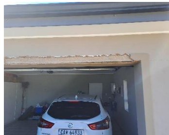
Pic 02: Cracks above lintel
