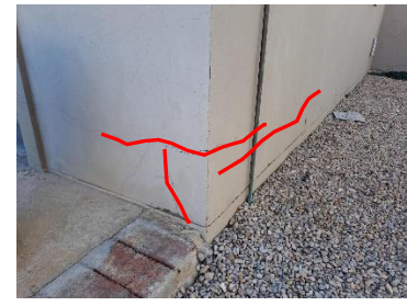
Pic 03: Cracks at corner brick wall
