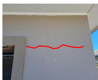
Pic 05: Horizontal crack on exterior and internal walls
