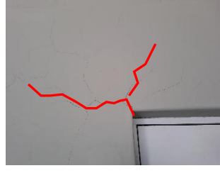
Pic 10: Crack above door leading into the kitchen
