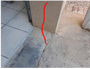
Pic 08: Crack in foundation continuing into exterior wall
