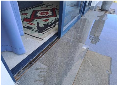
Pic 05: Standing water on the 1 st floor patio
