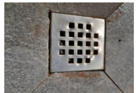
Pic 10: Poor waterproofing of the full-bore trap on the patio results in leaks to the living room
