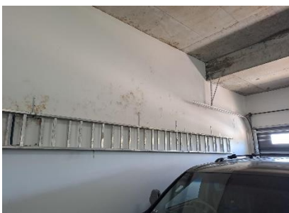
Pic 04: Water damp on the garage wall
