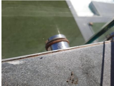
Pic 06: Tile edges not flush with tiles
