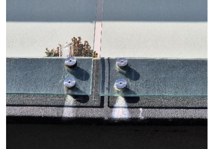
Pic 07: Water seepage - balustrade fixing bolts
