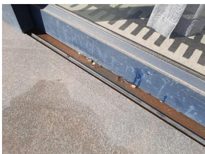
Pic 08: Water ingress into gaps between the sliding door rails and patio tiles
