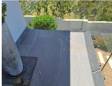
Pic 02: Water ingress in the patio tiles
