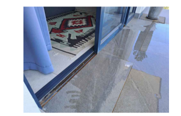
Standing water on patio sloping towards outside door opening
