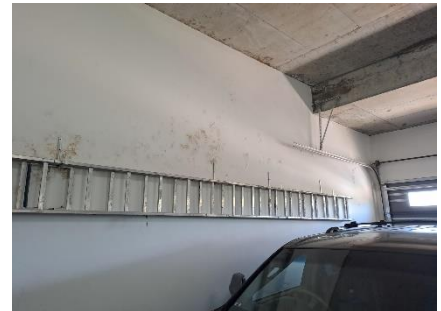
Pic 03: Water ingress on the garage walls
