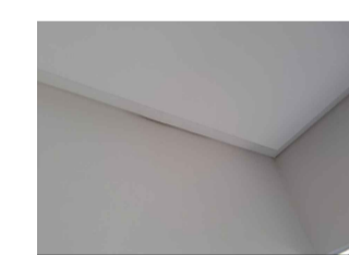
Water seeps into ceiling void in Living room
