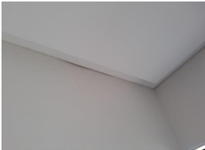
Pic 01: Water ingress from the 1 st floor roof
