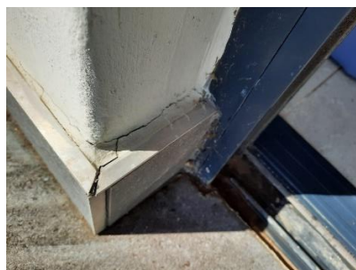
Pic 09: Blue coloured water seeping into cracks in walls and patio tiling
