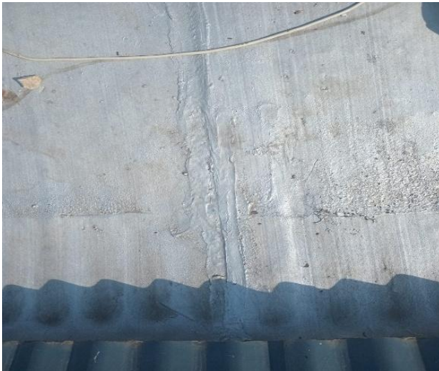
Figure 8: Protruding grooves on screeded surface 2
