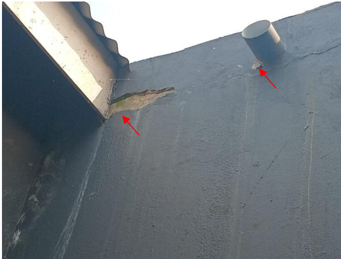
Figure 14: Water damage on external walls
