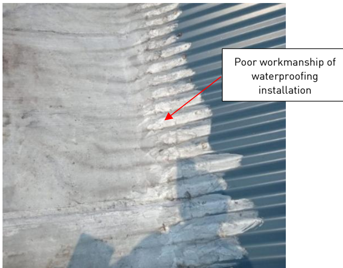
Figure 12: Poor Application of Waterproofing
