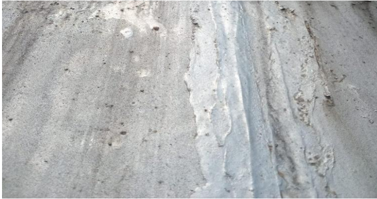
Figure 5: Protruding grooves on screeded surface 1
